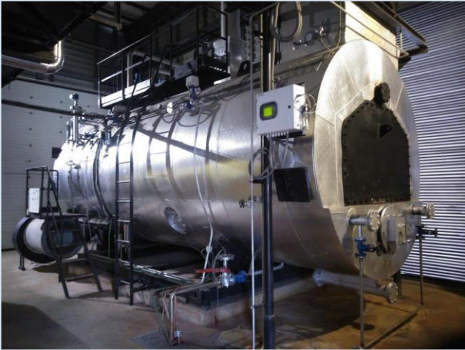
Prio’s 8 MW fire-tube boiler - 10-bar steam, fired by methane. 10-yr PPA · ~€5.7m saved.
