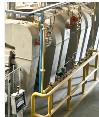
Primus gas-fired furnace, the process being replaced
